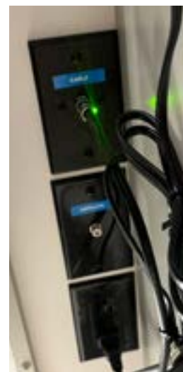
ANTENNA POWER SUPPLY
